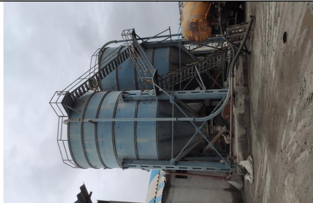
Fly Ash & Cement Feeding system
