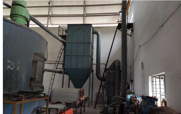
Fibre Dust Collection System
